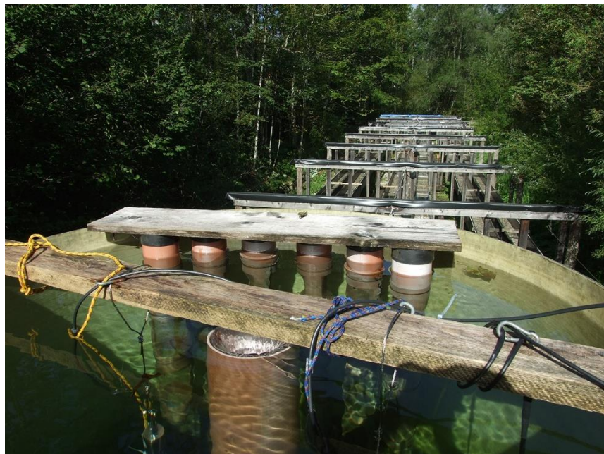
Header Tank with inflow pipes.
